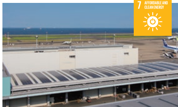
Installing solar panels on the rooftop of the domestic cargo terminal in Tokyo International Airport
